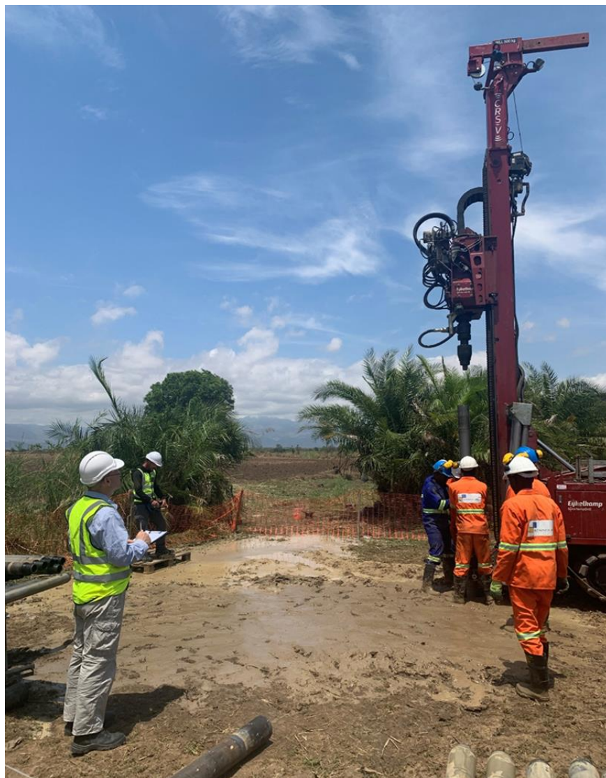
Figure 1 - The Competent Person, Mr Mark Burnett, from AMC was on site to review drilling procedures.
